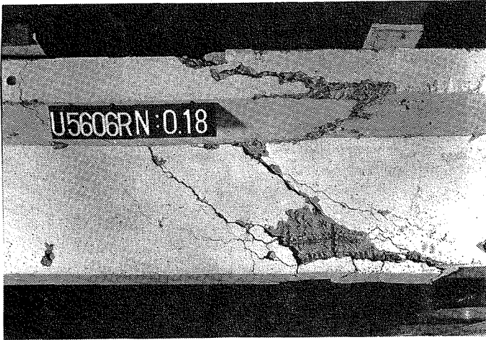
Fig.6.4: Fatigue failure of concrete struts. V_{\max} = 0.74 V_u
