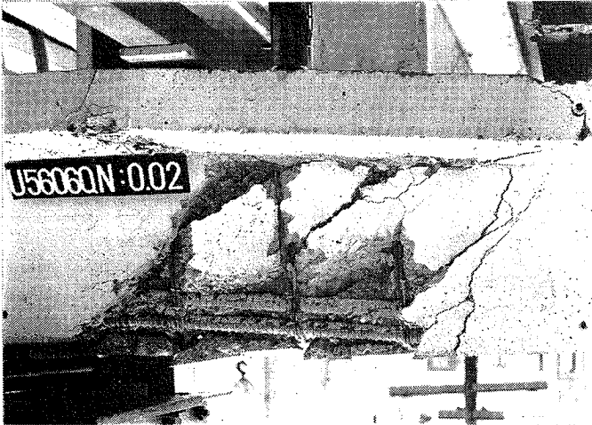
Fig.6.3: Fatigue failure of concrete struts. V_{\max} = 0.76 V_u
